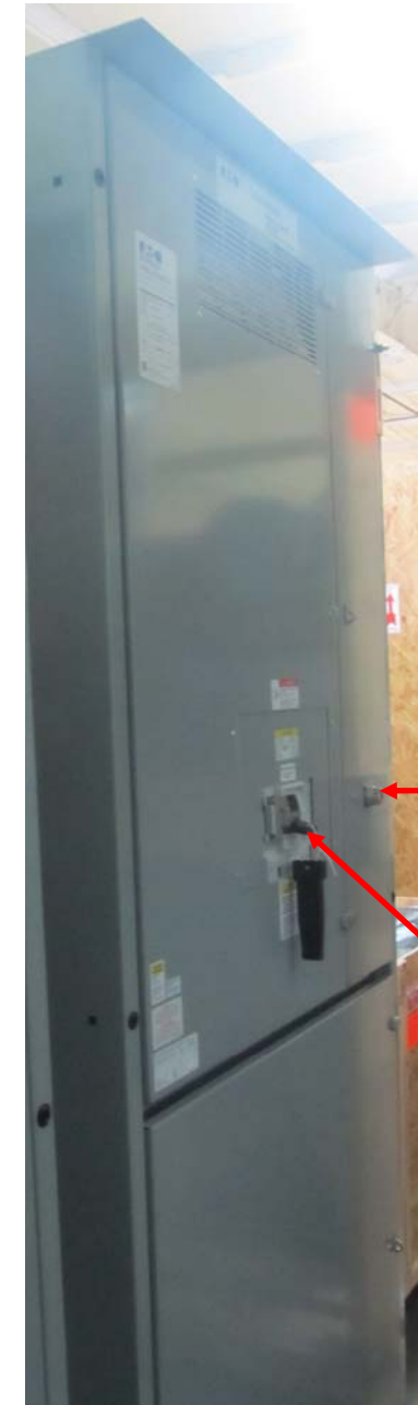
RIGHT-HAND CABINET (INPUT BREAKER)
