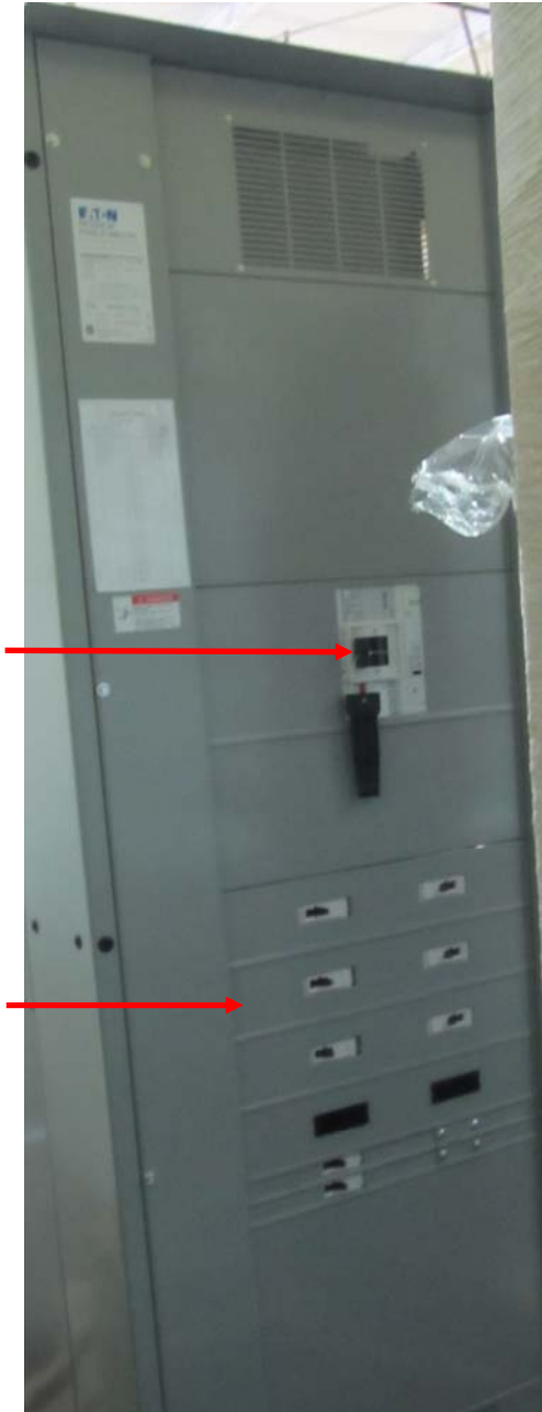
LEFT-HAND CABINET (OUTPUT BREAKERS)
