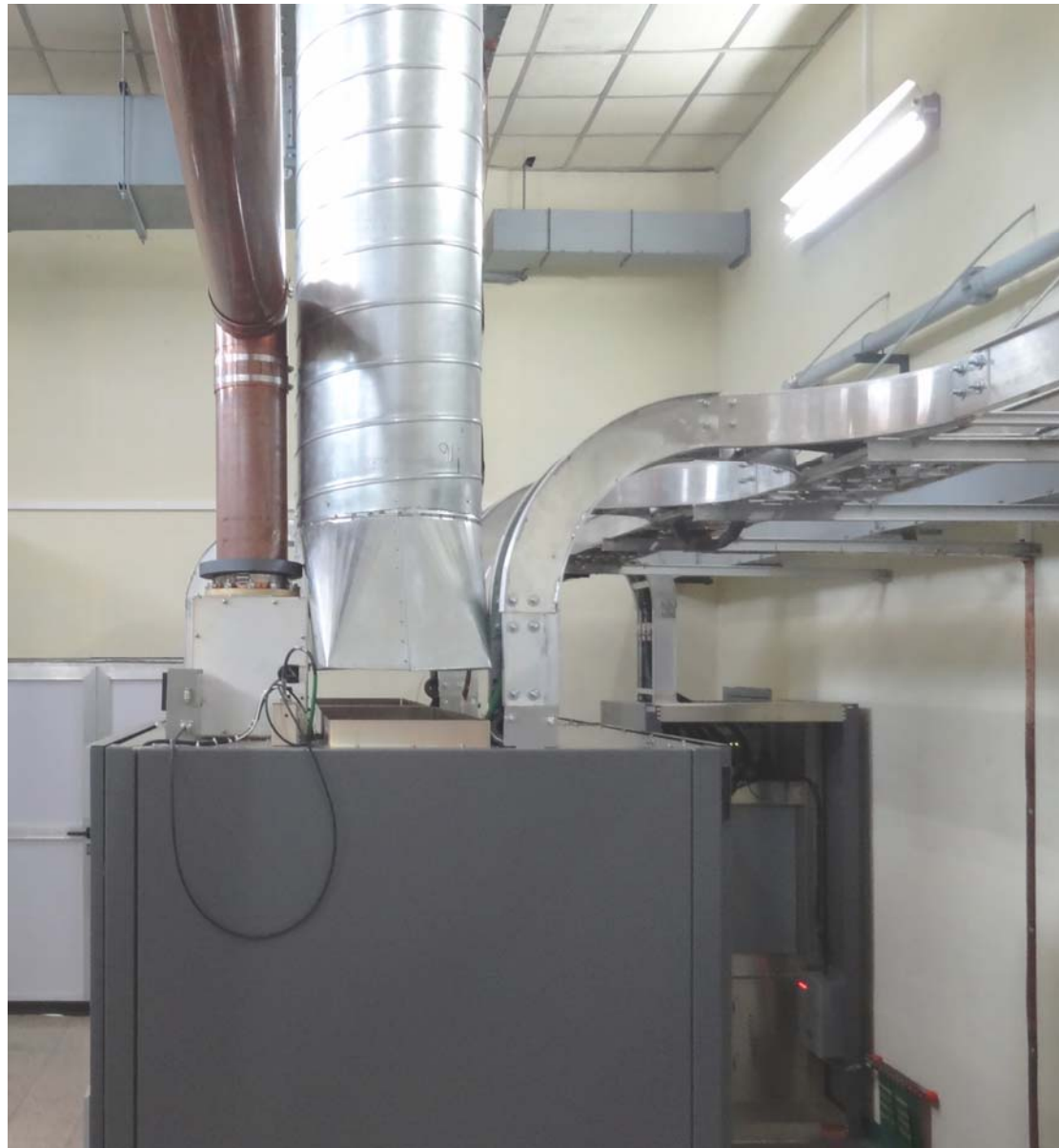
A Side View showing constrained area at top of NX300 transmitter.
