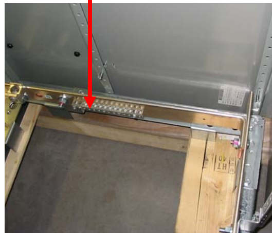
View of cabinet bottom
