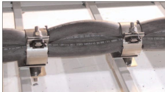
Properly restrained cables shown after a short circuit.
