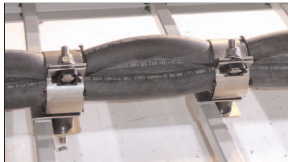
Properly restrained cables shown after a short circuit.
