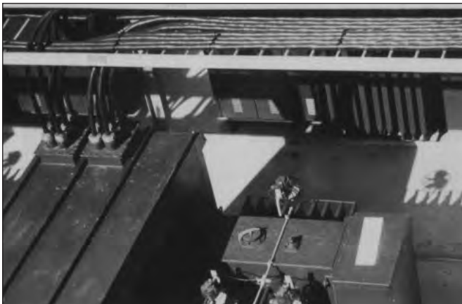
Cables Exiting 480 Volt Outdoor Switchgear and Entering Cable Tray System (Cable fittings with clamping glands are required to prevent moisture flow into equipment due to the cable's overhead entry into the switchgear enclosure).
